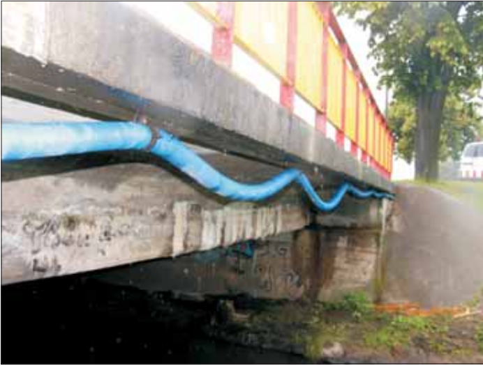
Fig. 3. Bridge side view – visible leakages of calcium carbonate on the side of the slab and on the abutment wall
