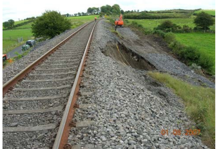
Slope failure near Castlebar Co. Mayo (2007)
