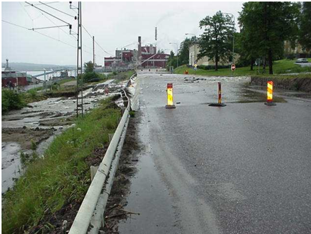
Figure 3: The road was flooded and damaged during a period of heavy rain in year 2000. (Photo, SRA).
